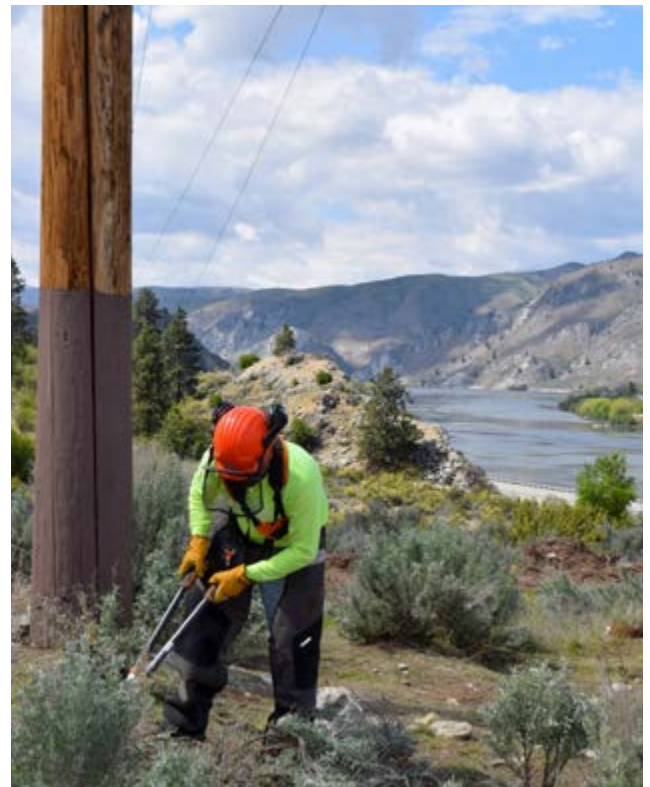
Climate change is projected to increase the risks of many extreme events, including wildfires. Chelan PUD grubs and paints poles as a proactive measure.
